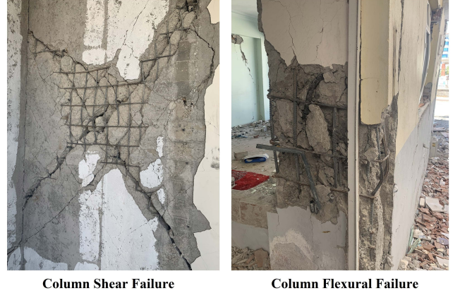
Figure 5: Reinforced concrete column failure modes in post-earthquake buildings considered in this paper
